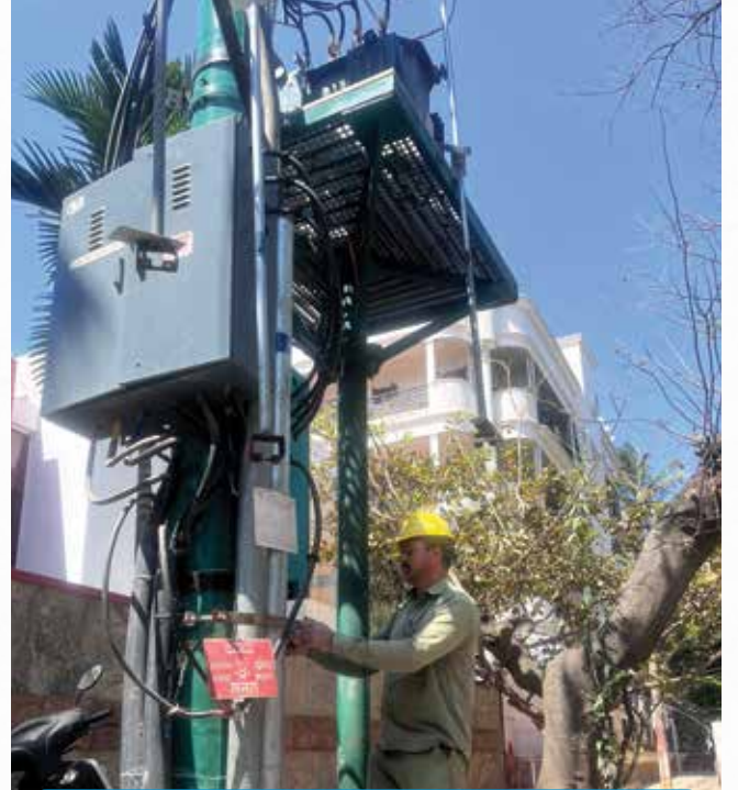
Traditional transformers replaced with specially designed Spun Pole High-Rise Transformers
