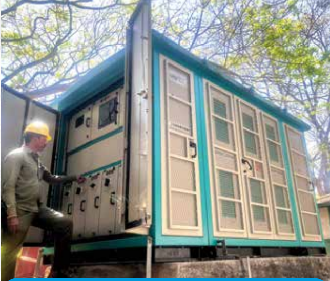
Transformers on footpaths replaced with Compact Transformers
