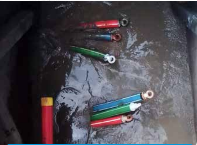
Three additional empty ducts provided to prevent road digging for future cable laying
