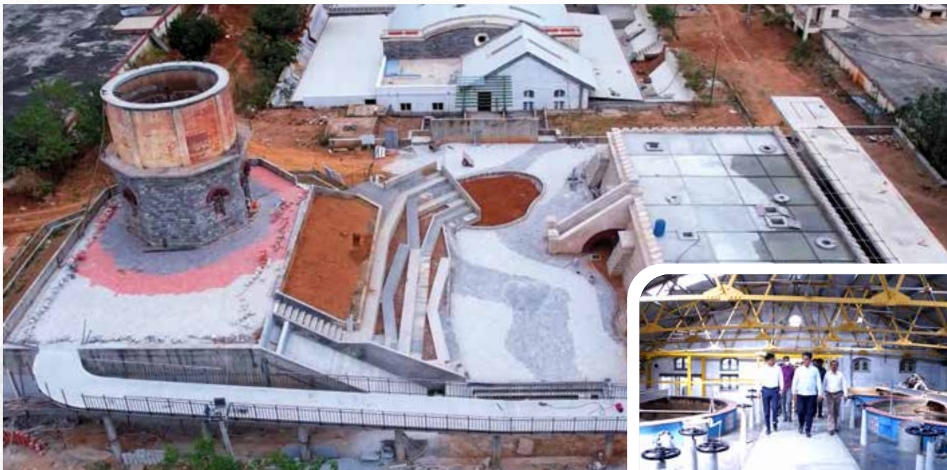
BWSSB Museum comprising Pump House, Museum & Central Plaza being setup. Will help raise awareness on effective water management
